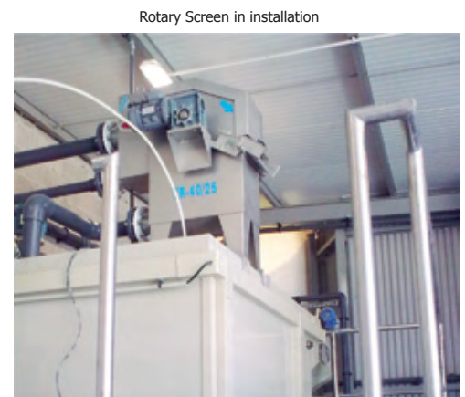
Rotary Screen in installation
